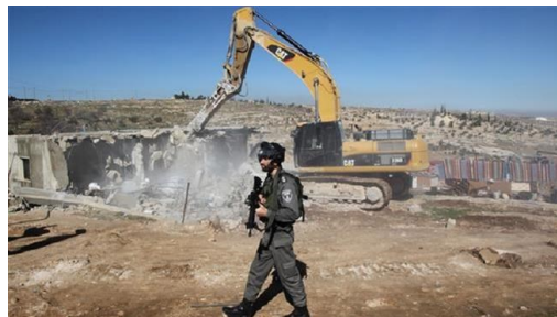
Israel has demolished more than 48,000 Palestinian buildings in the occupied territories since 1967
